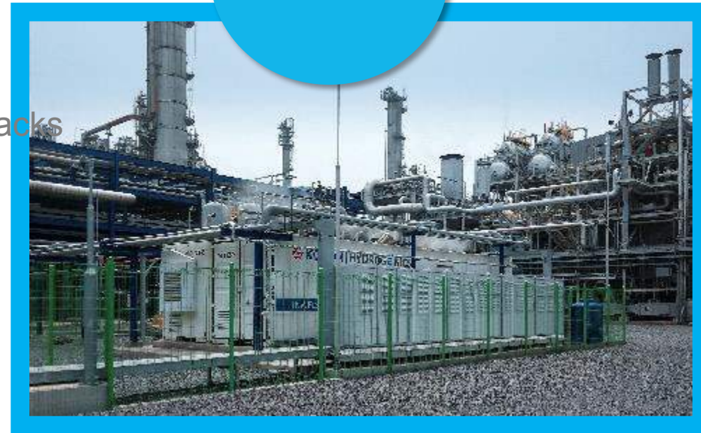
1 MW Stationary Fuel Cell Plant
